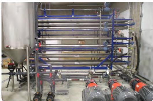
The IUH can treat five million gallons of wastewater a day within 15,000 square feet
