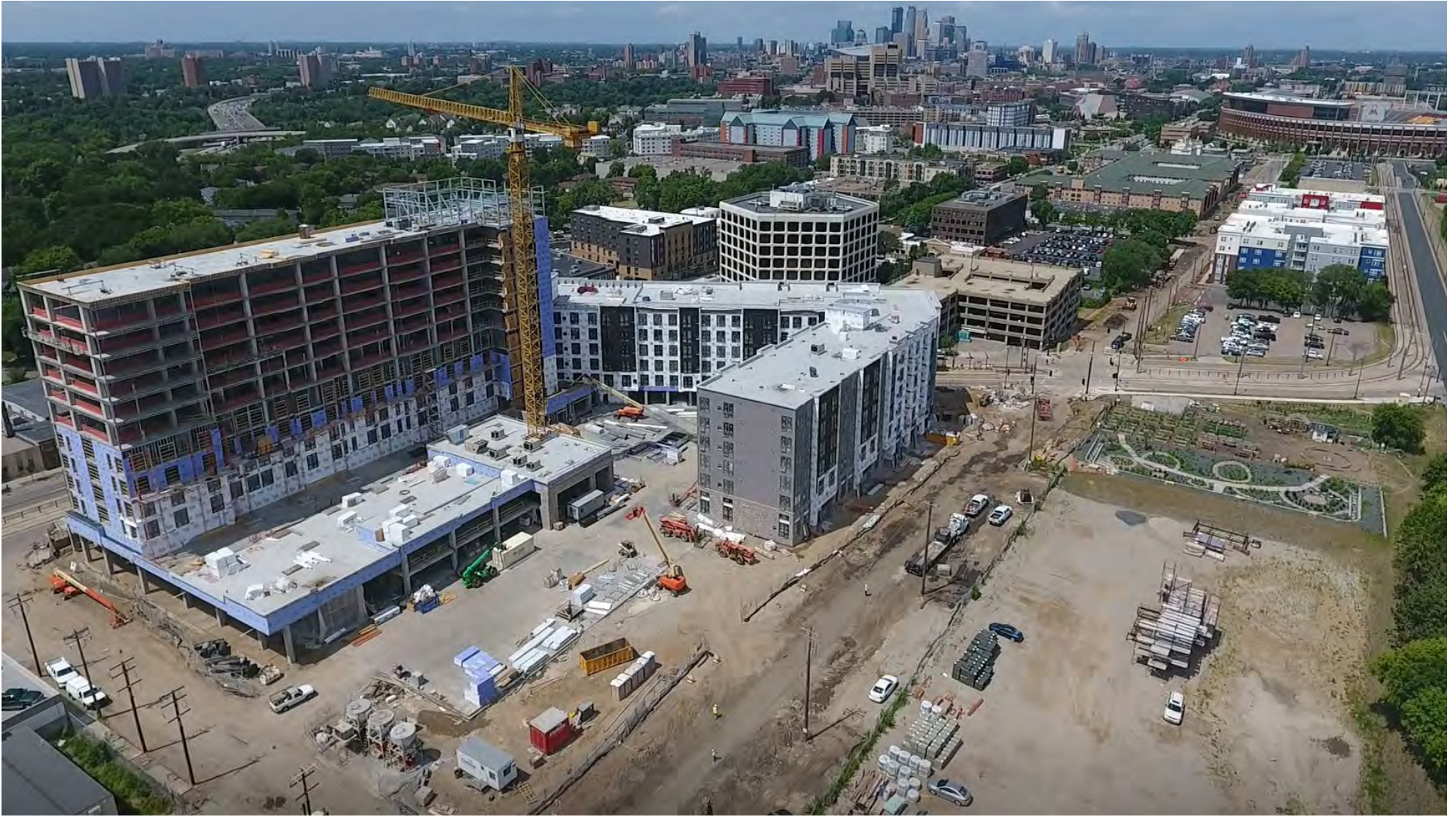
Construction of a major housing and mixed use project at Towerside—The Link.
